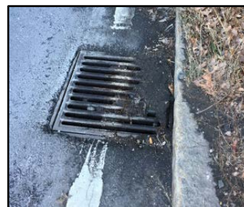
Image 7: Debris within Dascomb Road catch basin.
