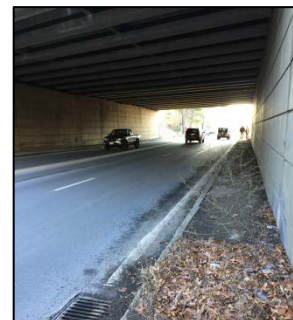
Image 3: Debris located on sidewalk below I-93 overpass.
