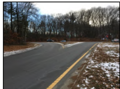
Image 5: Lack of YIELD signage and markings on Dascomb Road channelized lane.
