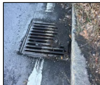
Image 7: Debris within Dascomb Road catch basin.
