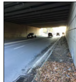
Image 3: Debris located on sidewalk below I-93 overpass.
